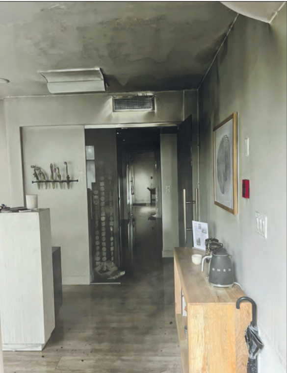
The Woods Arts & Wellness is facing extensive smoke and water damage after a fire broke out in one of their counselling rooms. EMILY THOMPSON
